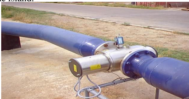
Figure 8: UV installed at the discharged pumped of the storage tanks at W.E.B. ARUBA N.V.
